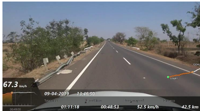
Broken crash barrier Km 42.5, SH-20
